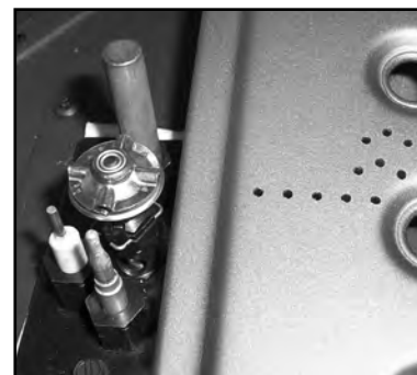
Figure 8. Ignitor assembly beside the burner.
