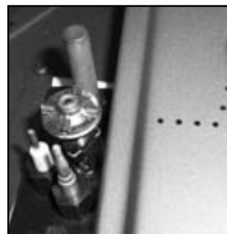
Figure 9. Ignitor assembly beside the burner.
