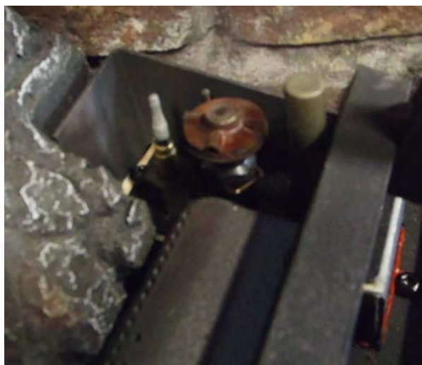
Figure 15. Pilot assembly beside the burner.
