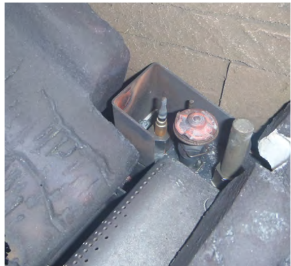
Figure 15. Pilot assembly beside the burner.
